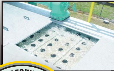
Hot Water Basins
