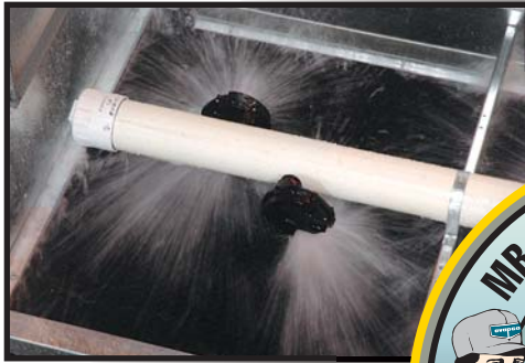
Water Distribution Systems
